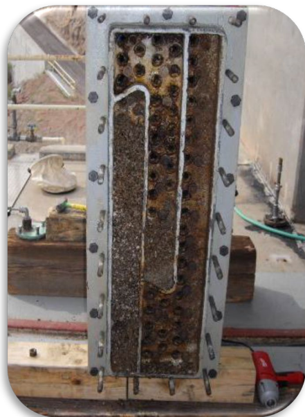
CAP Cooling Water Heat Exchanger
