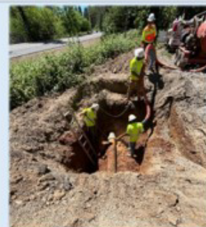
Master Meter Installation
