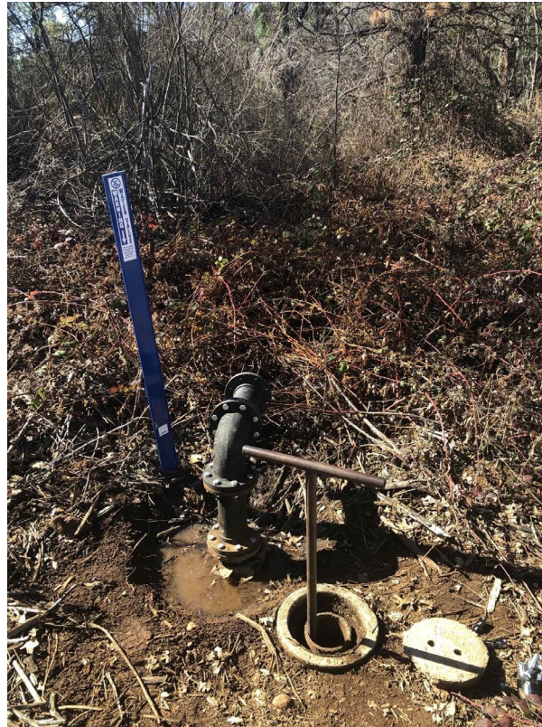
Blow Off Valve
